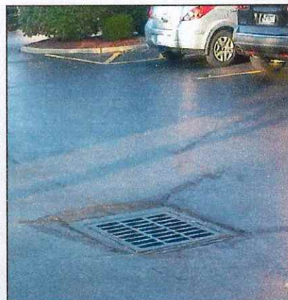
Runoff from coal-tar-sealcoated pavement goes down storm drains to receiving water bodies. The runoff contains high concentrations of PAHs and related chemicals that can harm aquatic life. 16
