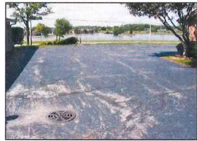
Light gray patches of asphalt show where sealcoat has been worn from the pavement. Applicators recommend reapplication of sealcoat from every 1 to 5 years. 1
