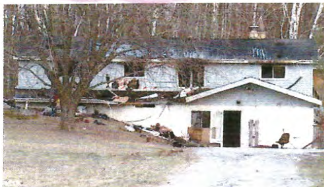
This home on Hwy. 141 in the town of Amberg was destroyed by fire, Nov. 27, 2013. (Photo from: FOX 11).
