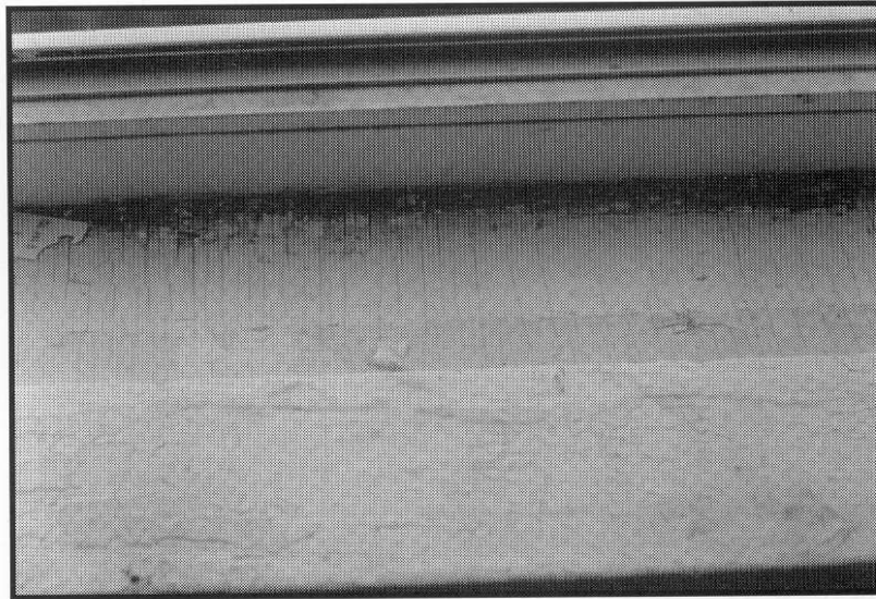
Figure 11.14a Turning a Window Sill and Trough Into a Smooth and Cleanable Surface (before treatment).
