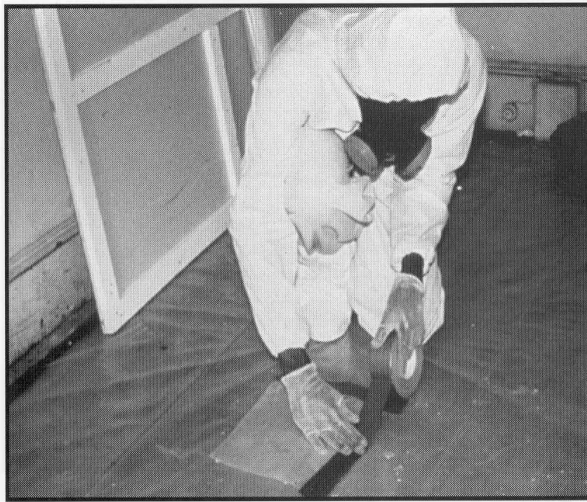
Figure 14.7 Plastic Sheeting Should Be Repaired as Part of Daily Cleanup.
