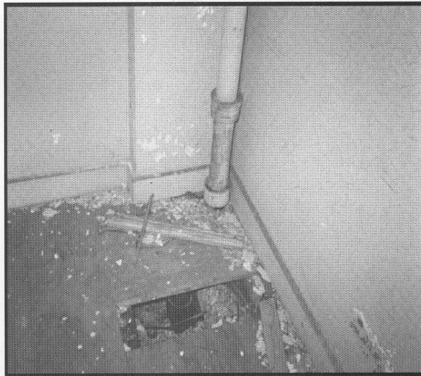
Figure 8.2 Area Should Be Precleaned and Structural Deficiencies in Flooring Repaired Before Lead Hazard Control Begins.
