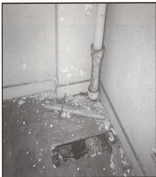
Figure 14.6 Pre-cleaning Is Needed in Areas Where Contamination and Deterioration Are High.
