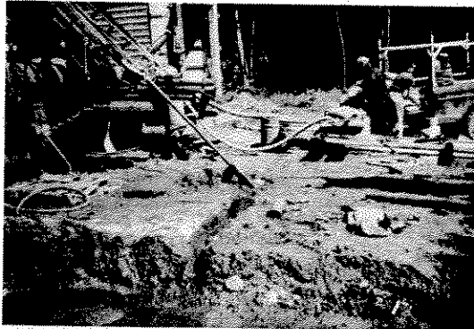
For this exploratory drilling in northern Wisconsin, the drilling mast is placed at an angle to permit the recovery of samples from rocks that are tilted below the ground surface. Exploration is regulated under ch. NR 130, Wis. Admin. Code.
