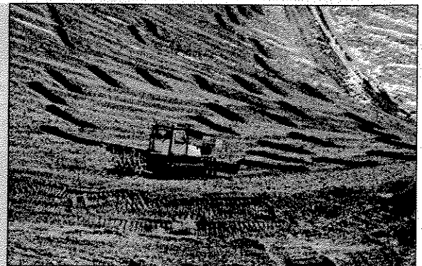
Left: Initial reclamation involved regrading to a 2V:1H slope with diversion ditches every 200 vertical feet.
